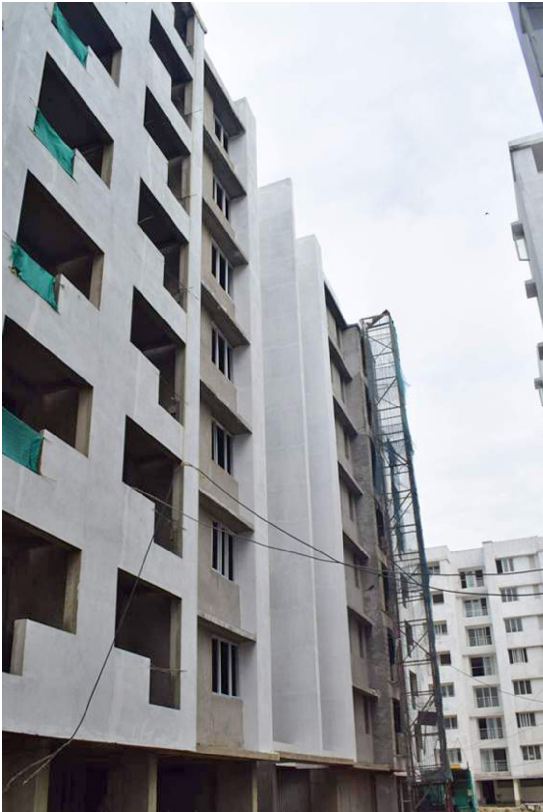
D15 Block - Internal wall Plastering works under progress, Water proofing in toilet - completed
