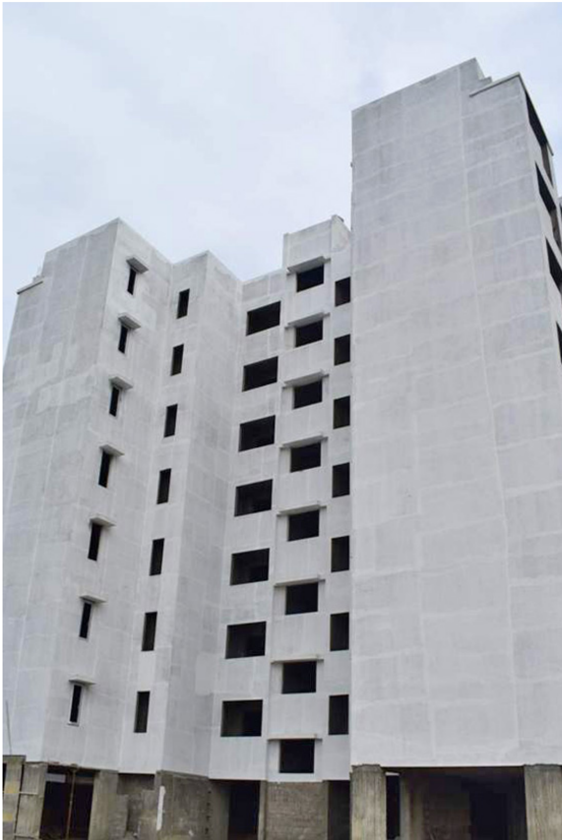
D14 Block - Internal ceiling plastering completed, Water proofing in toilet work in progress
