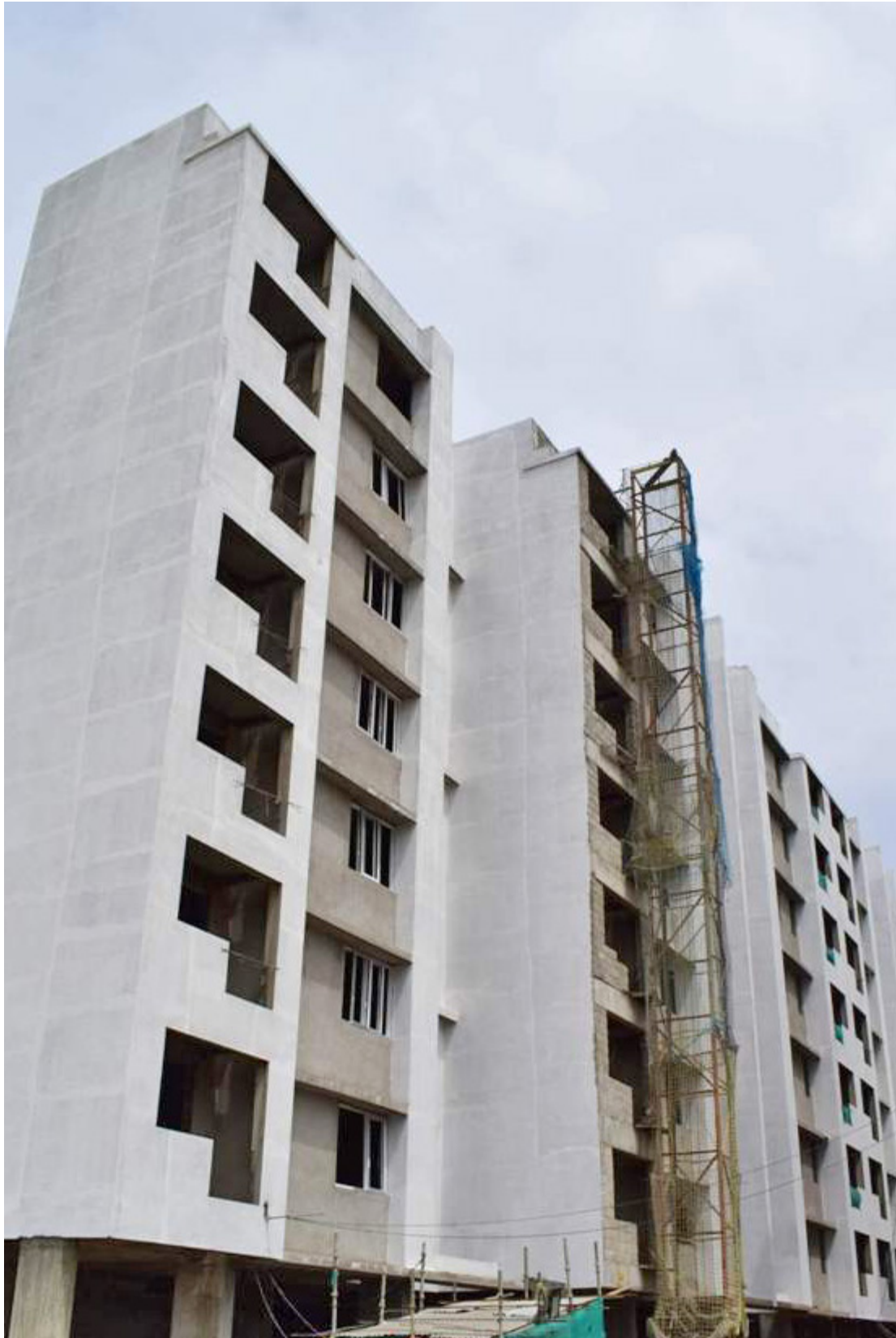
D14 Block - Internal ceiling plastering completed, Water proofing in toilet work in progress
