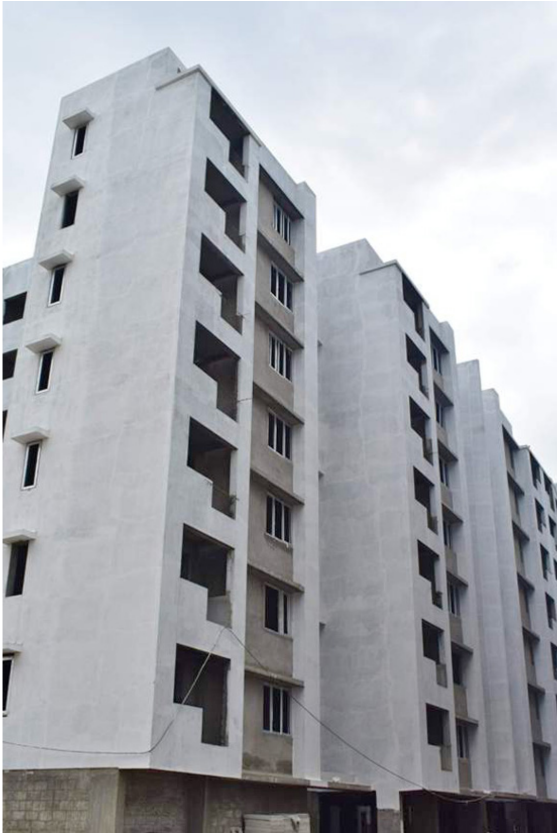
D15 Block - Internal wall Plastering works under progress, Water proofing in toilet - completed
